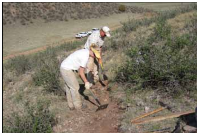
Constructing the Bent Rock Trail, Larimer County Trails and Projects Crew. Photo: Elijah Miller
